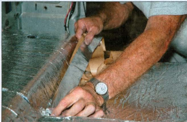
All seams were then sealed with aluminum tape to further isolate heat and keep any moisture from getting in under the Heat Shield.
